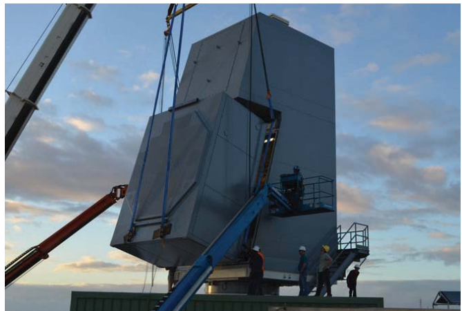
A crane lifts the Air and Missile Defense Radar into place for its upcoming tests at the U.S. Navy Pacific Missile Range Facility. (Raytheon)
